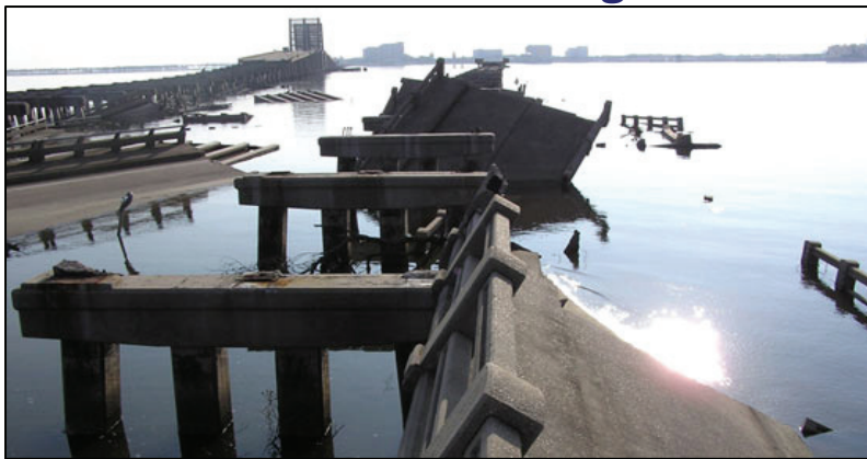
Damaged U.S. 90 Biloxi Bay Bridge after Hurricane Katrina (photo courtesy of Robertson, Yim, and Young).
